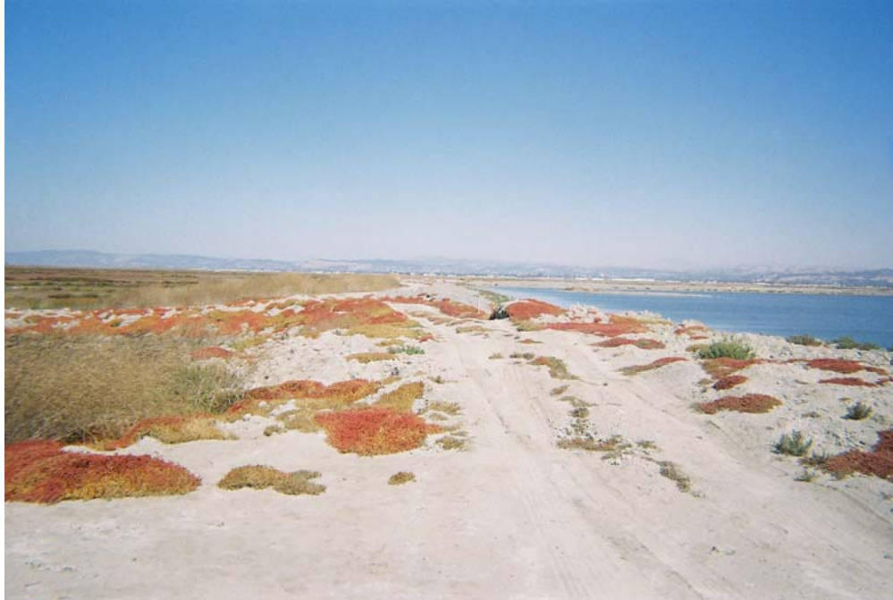
Photograph 7: Example of previous breach and overtopping distress of levee with subsequent poor repair (Pond B2 West)
