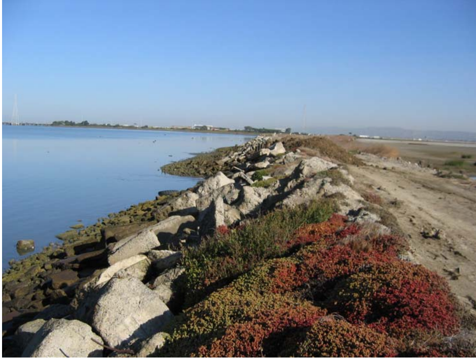
Photograph 3: Example of levee with broken concrete slope protection (Pond B10 West)
