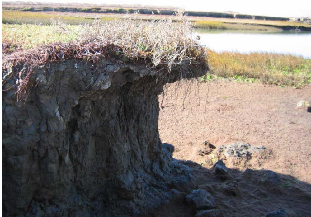
Photograph 8: Example of undercutting and severe erosion distress of levee slope (Pond BT1 Southwestern point)
