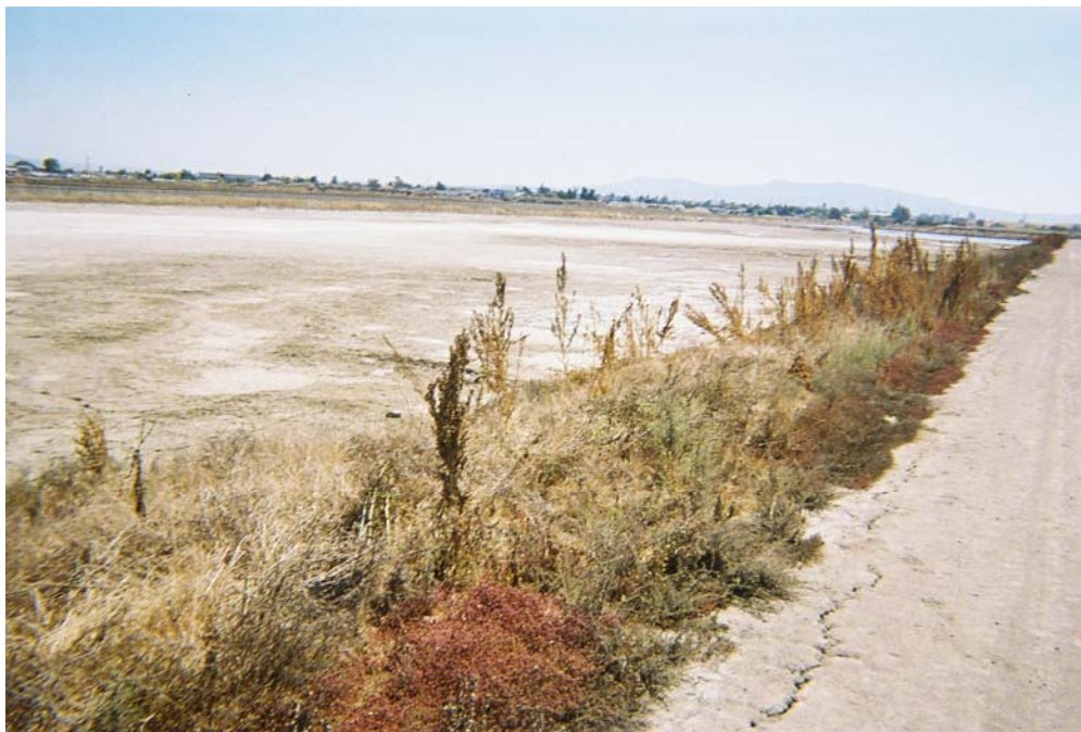
Photograph 6: Example of cracking distress of levee crest (Pond A12 East)
