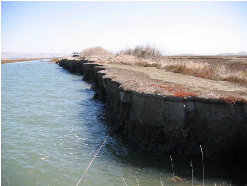
Photograph 10: Example of severe erosion distress of levee slope and crest (Pond BT2 North)
