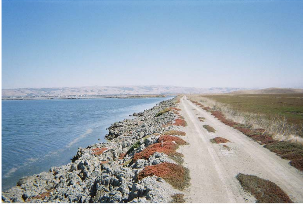
Photograph 9: Example of gullying and severe erosion distress of unprotected levee slope (Pond B2 South)
